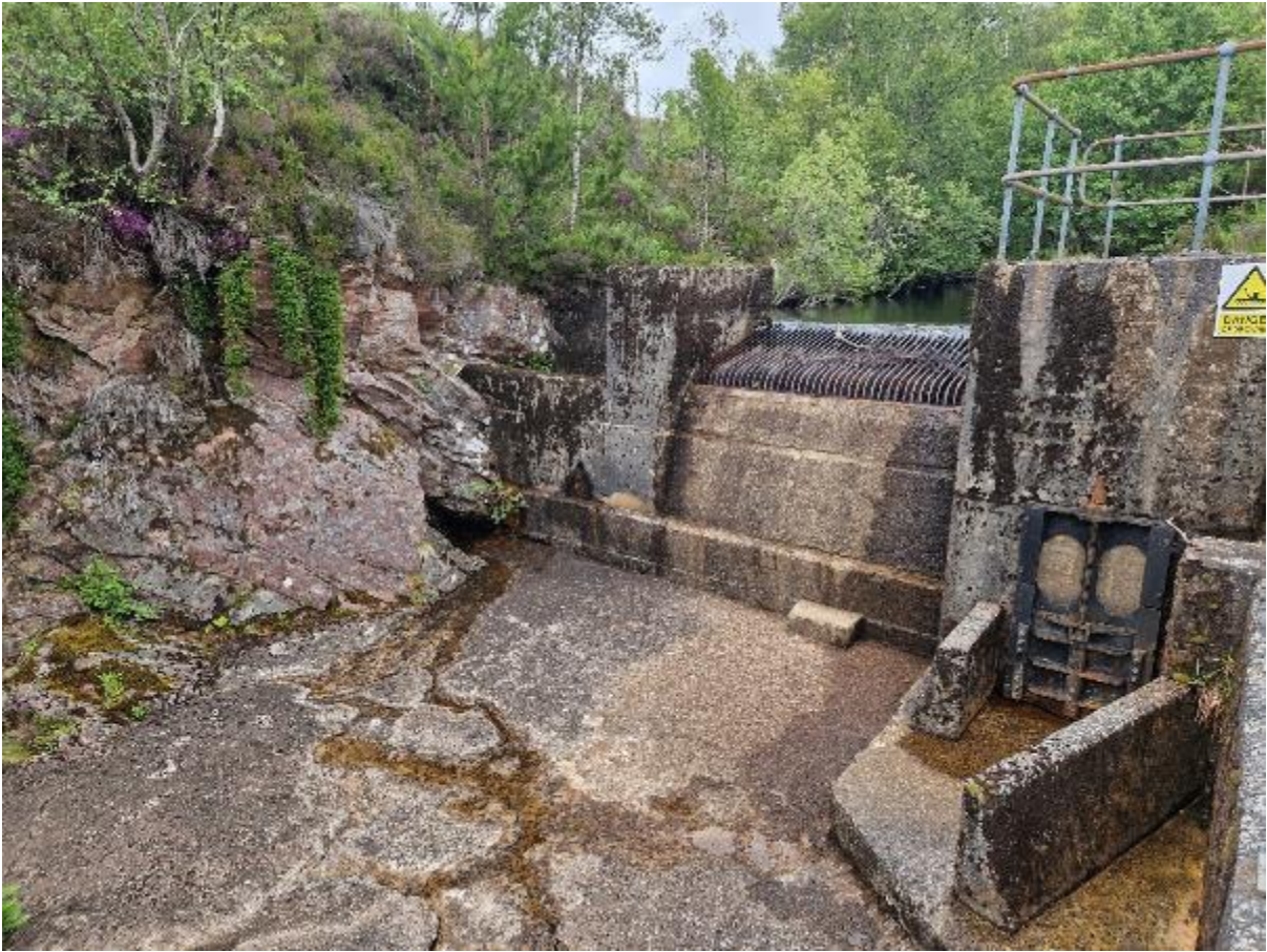
Figure 61: SSE Hydro intake structure at the lower end of the survey area.
